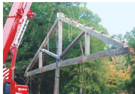
Lifting one of the truss' off the ground, ready for bolting to the framework
